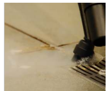
Tiles and Grout
