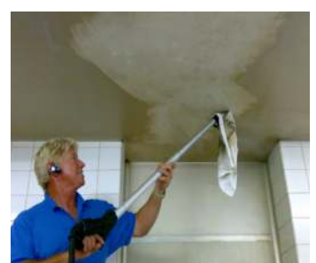
Heat Stains on Ceilings
