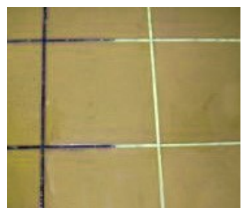
Tiles and Grout
